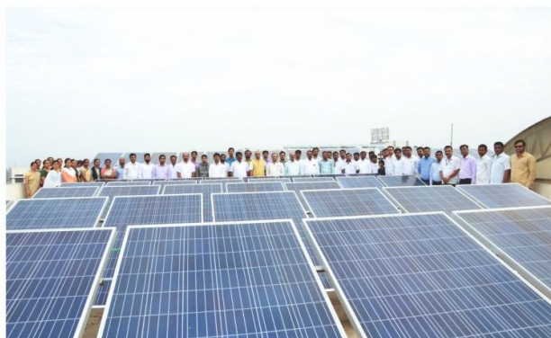
Solar Power Generation Plant (70 KVA)
