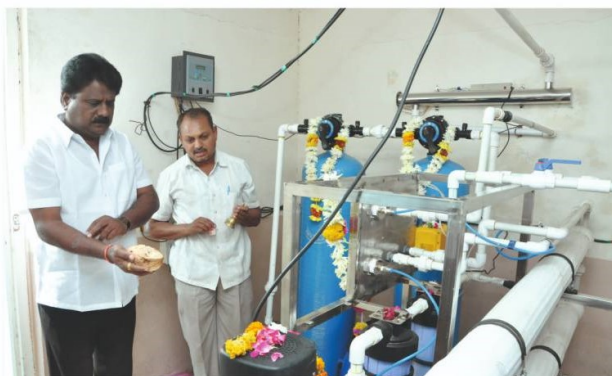
RO / UV Water Purification Plant
